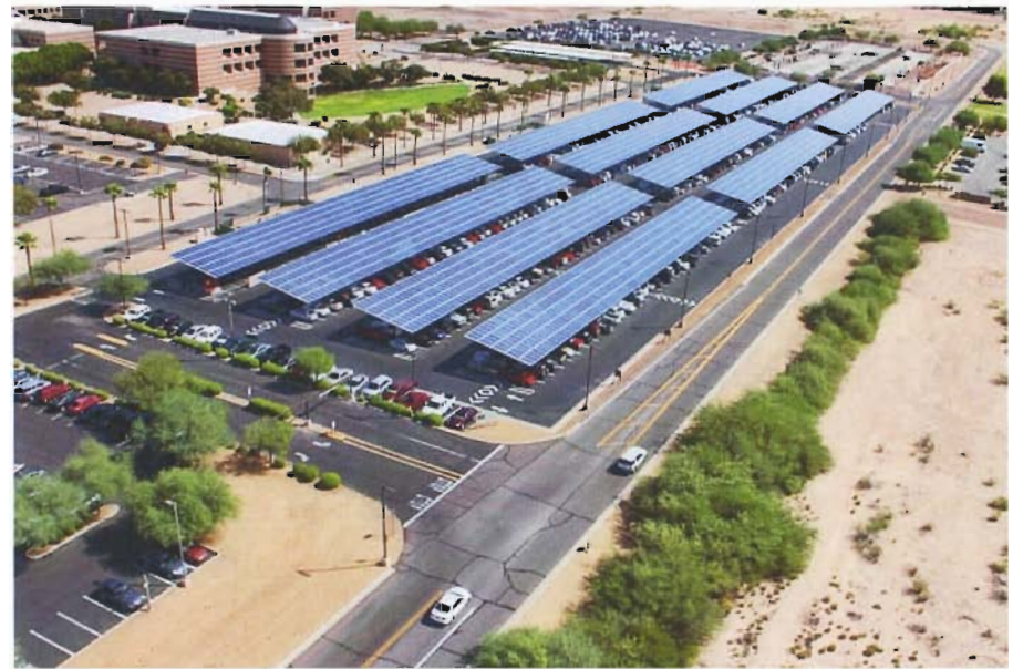
Arizona State University West Campus Carports – 1.2 MW
